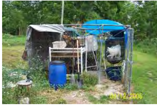
8-20. Shelter (dog) not structurally sound 3.1(a)
